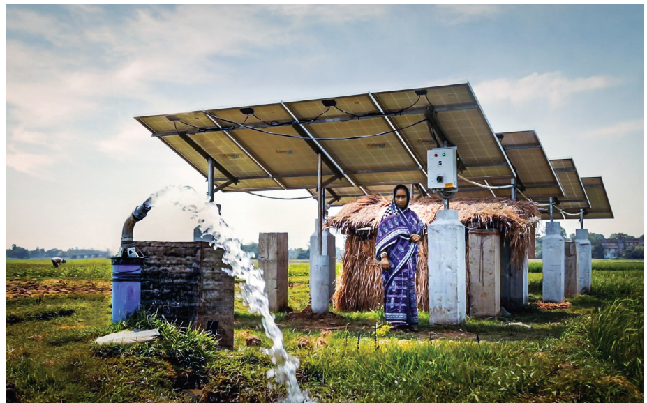
Alpana Pal, a beneficiary of solar pump installation at Mongolkote, Purba Bardhaman district WB
